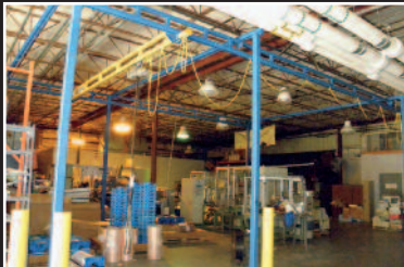
Gorbel Bridge Crane System
