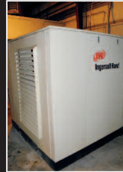
Numerous Ingersoll Rand Rotary Screw Air Compressors
